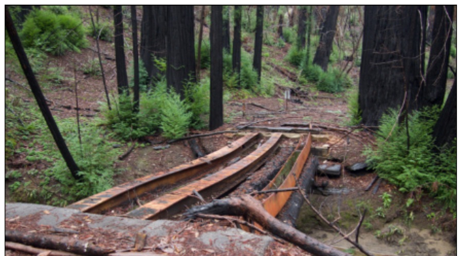
The last bridge over Opal Creek had been destroyed. The steel I beams were left, sagging from the heat, revealing the old redwood log stringers.
